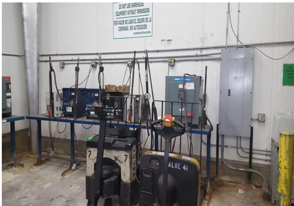
Photograph 14: View of the forklift charging area on the eastern side of the building
