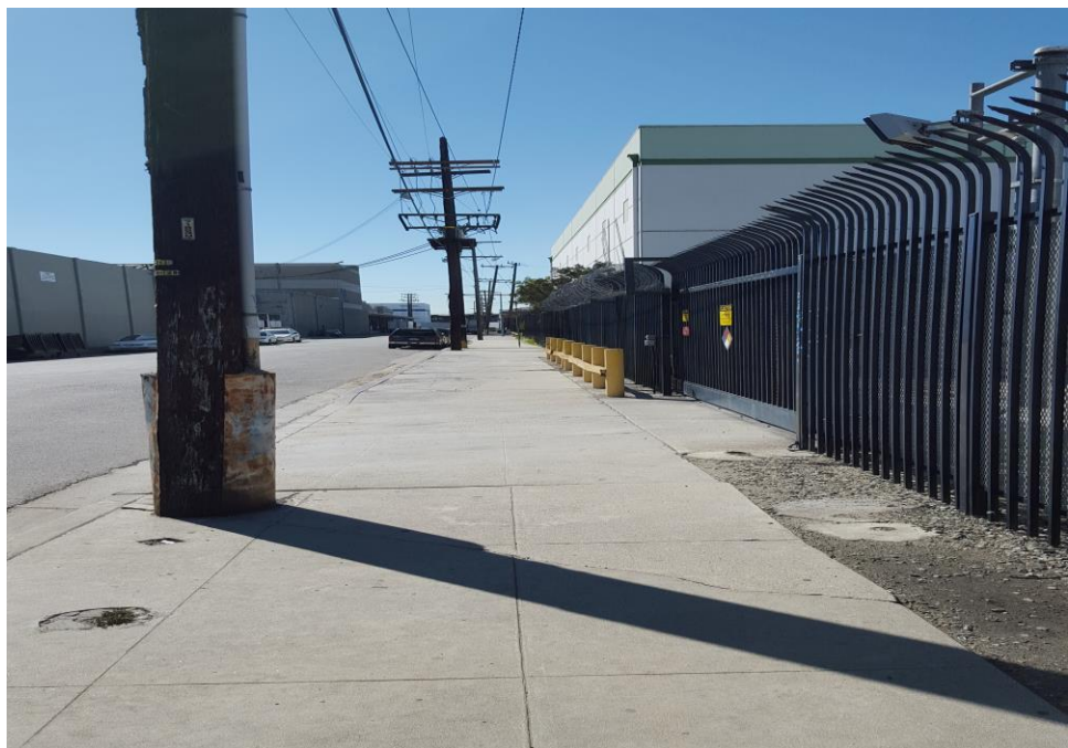
Photograph 10: View of the pole mounted transformers adjacent to the northwestern boundary of the site.
