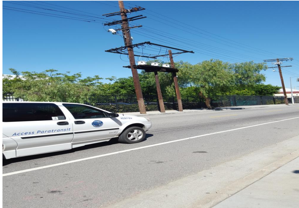
Photograph 11: View of the pole mounted transformers across the street, west of the site.
