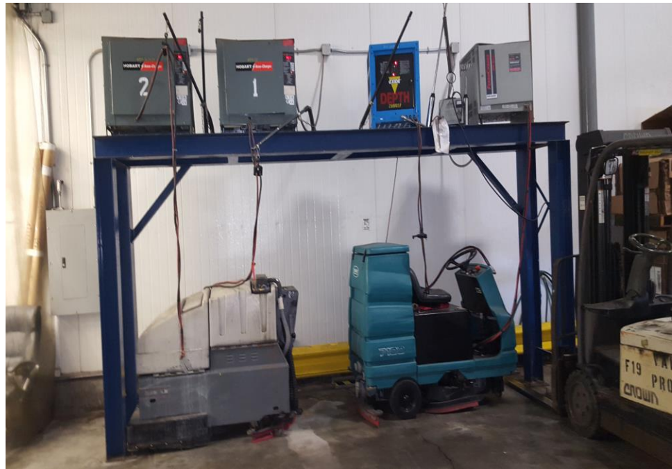
Photograph 15: View of the forklift charging area, and storage area of industrial cleaning machines on the western side of the building.
