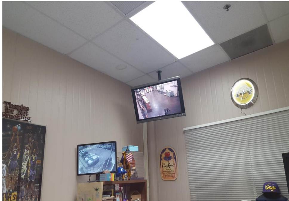
Photograph 19: View of water damage on the ceiling of office on the western portion of the building.
