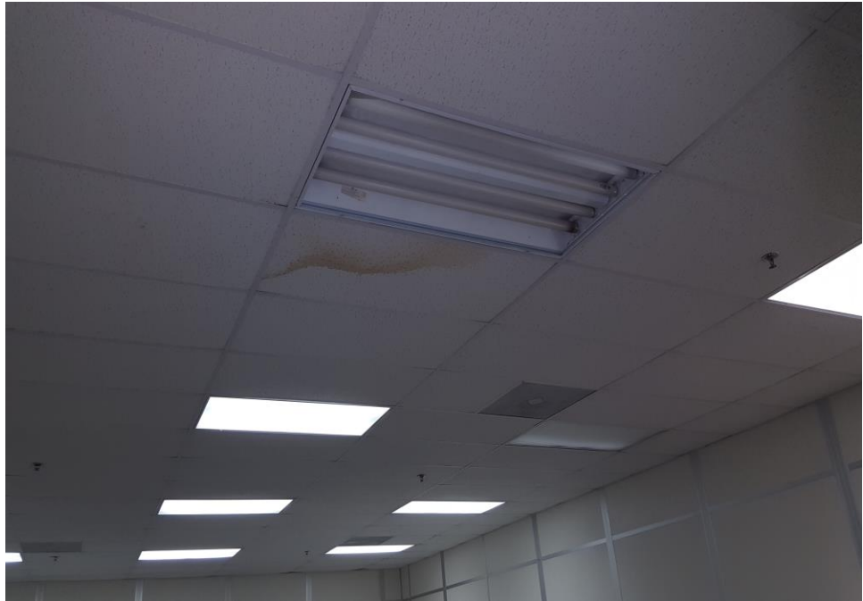
Photograph 21: View of water damage on the ceiling of office on the eastern portion of the building.
