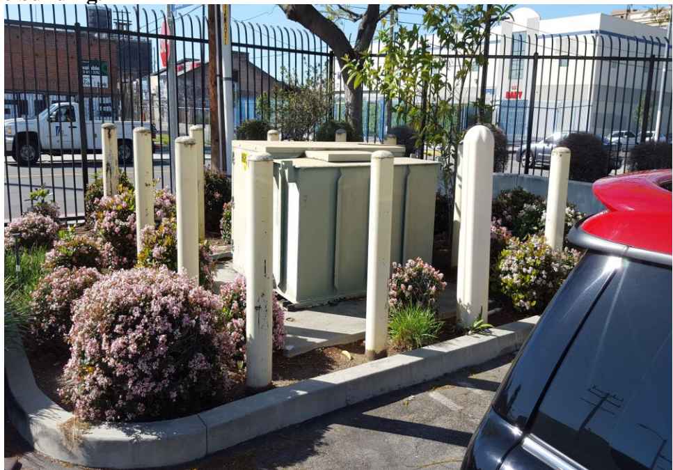
Photograph 22: View of the transformer on the southwest corner of the parking lot.
