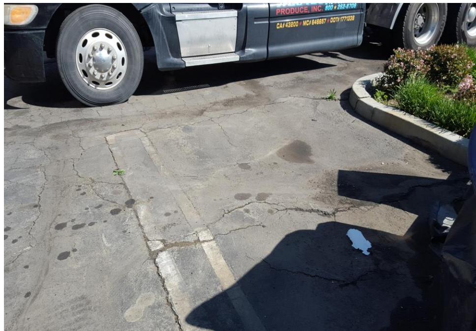
Photograph 24: View of stained and cracked concrete on the eastern portion of the parking lot.
