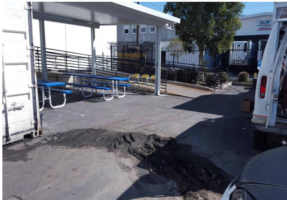
Photograph 26: View of asphalt section in bad condition on the eastern portion of the parking lot.
