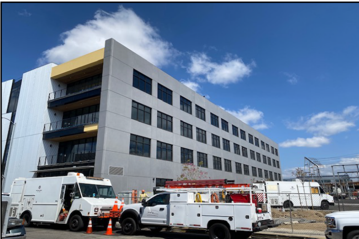
View 5: On the southern side of Jesse Street, looking northwest at the Project Site.
