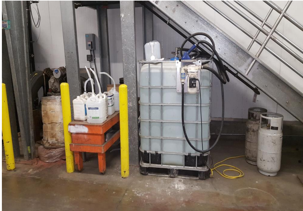
Photograph 13: View of 200-gallon DEF AST, unknown powdery substance in a 55-gallon drum and two propane tanks located on the southeast portion of the building.
