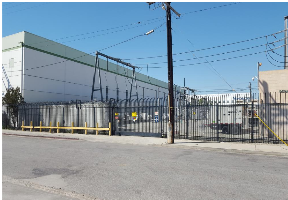
Photograph 6: View of the Los Angeles Department of Water and Power LADWP, Generation Station adjoining property to the north of the site.
